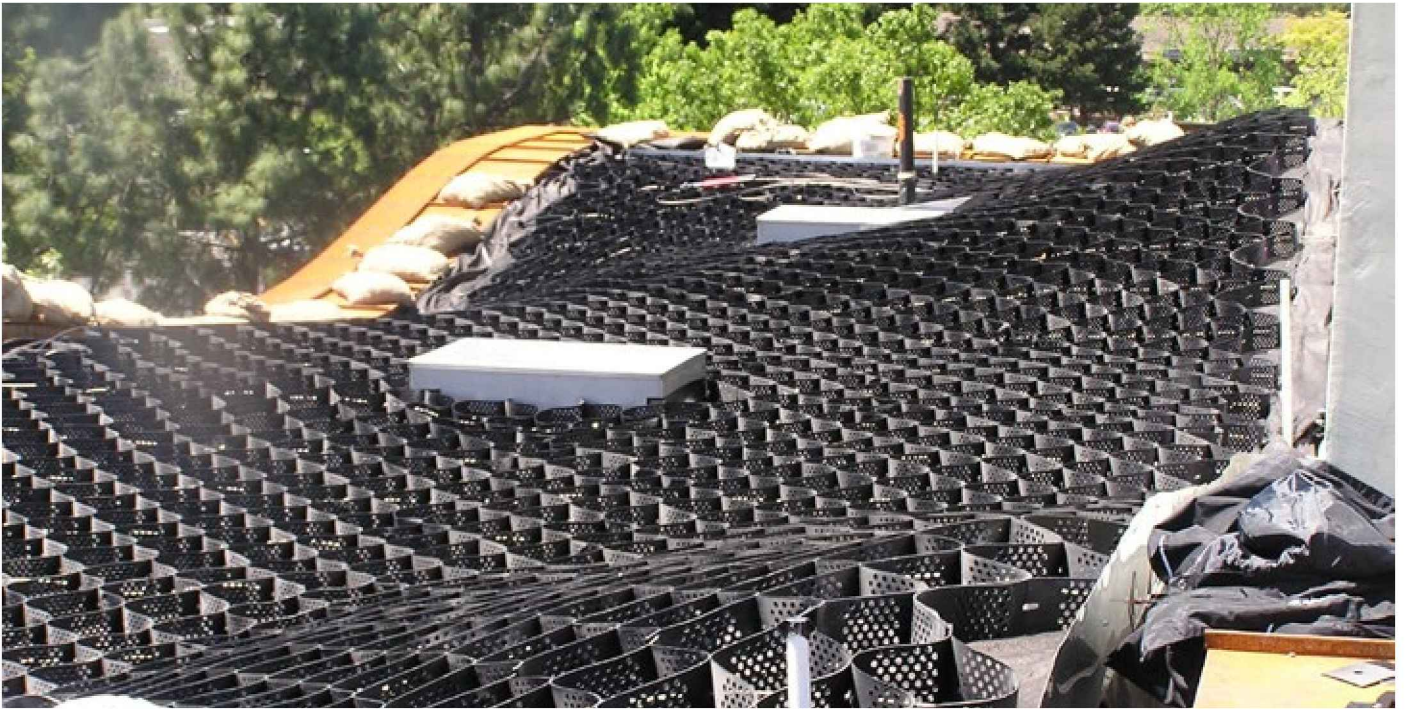
This unique green roof at the H2Hotel was created using stacked DuPont Styrofoam.
