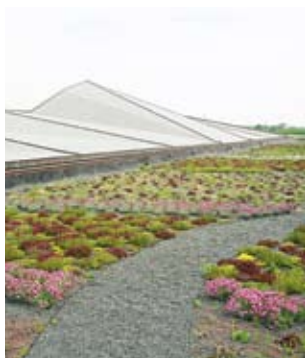
An extensive green roof tops Oak Park Library, Oak Park, Ill. Photos courtesy of American Hydrotech.
